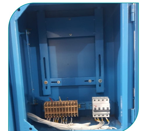
MCB METERING BOX IN DTR'S
