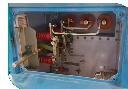
HV DRY TYPE ISOLATOR CONNECTION IN DTR
